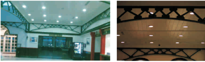
Picture of lights installed in Overseas Chinese Town (OCT)
